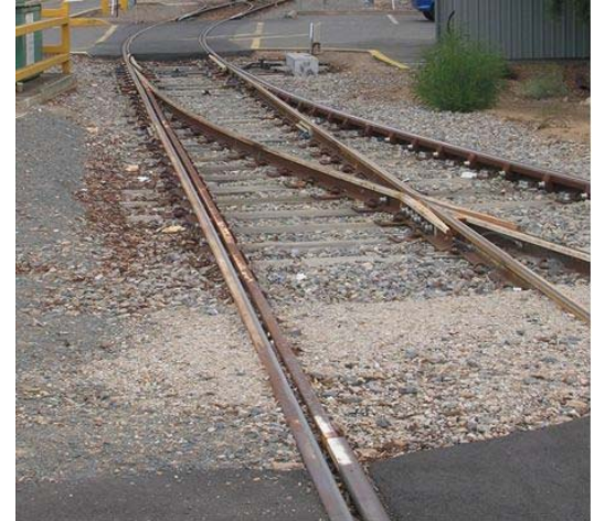
Figure 25 – Turnout 9A after One Year of Operation
