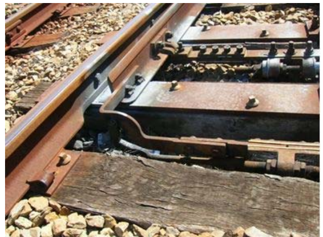
Figure 14 – 60kgAS Bevel Undercut Switch at Wye Cabin
