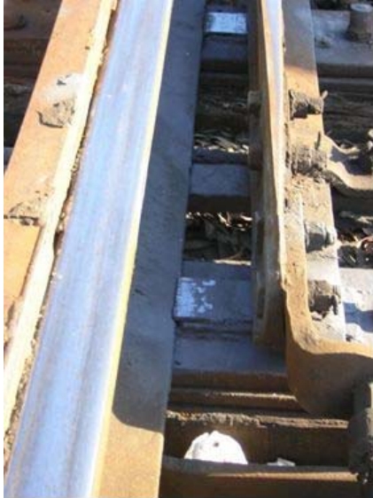
Figure 6 – Broken Point of Blade and External Checkrail
