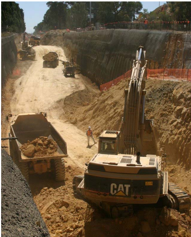
The cutting past Box hill cemetery looking toward Box Hill on Mon 8 th Jan. The original track level was near the surface at this point (perhaps 2 metres deep). Spoil was removed so quickly that it was stacked on Box Hill High School oval for later removal, rather than tie up the actual work by carting it away as it was dug out.
