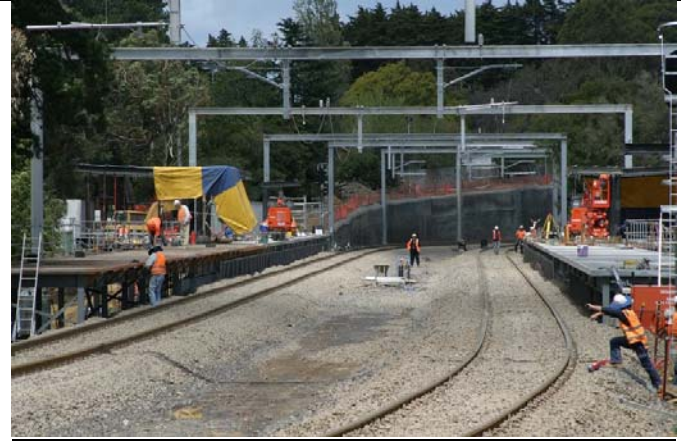
New Laburnum station looking toward Box Hill showing the start of the cutting which replaced the 1 in 40 grade and allowed Middleborough Road (around the corner to the right) to go over the top. The future third track will go down the middle.
