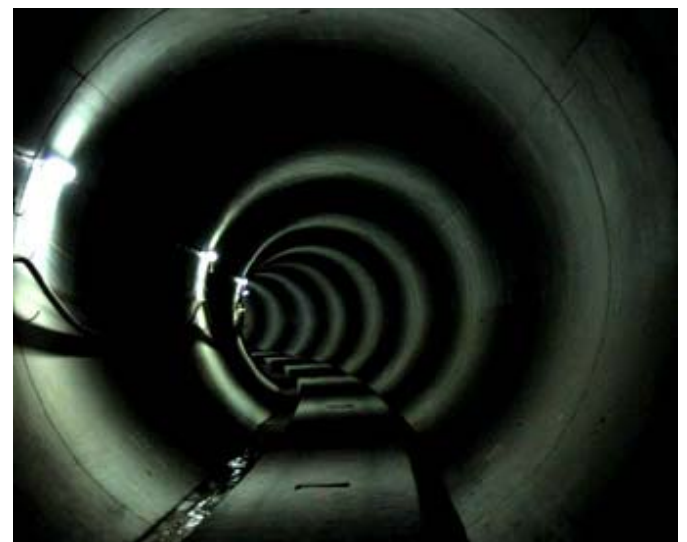
The inside of a tabby cat? No, the completed tunnel looking toward Chatswood.
