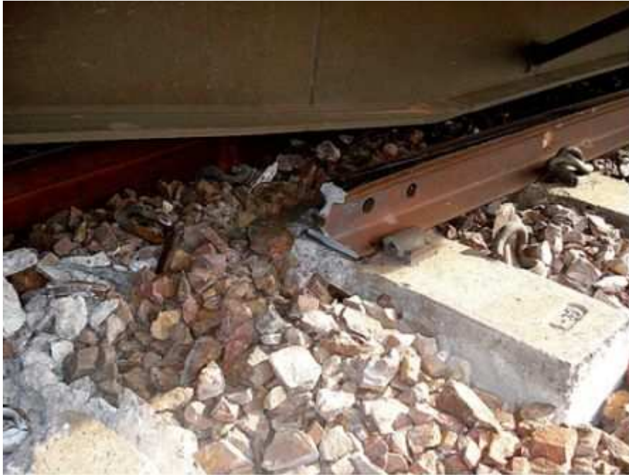
Broken Rail. (The cause of this derailment)
