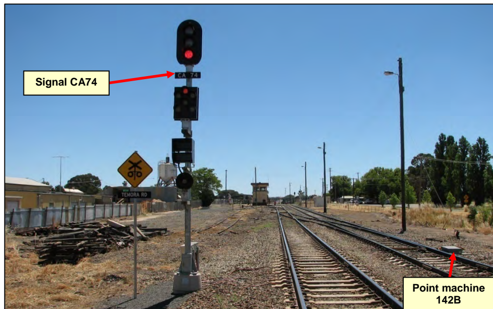
Figure 5: Typical items of field hardware – Signal CA74 and point machine 142B
