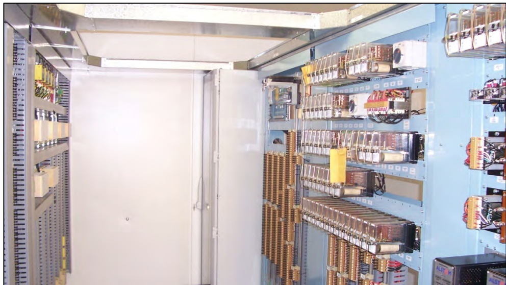
Figure 6: Typical Microlok relay room
